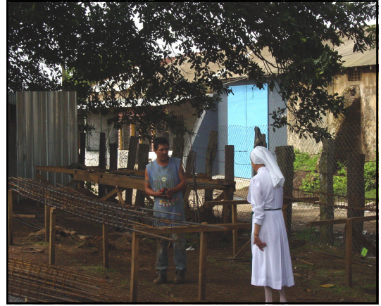
Sister Claudia Fernandez , Hospital San Jose, Diriamba, Carazo, in the midst of a major Hospital expansion project chats with an employee on the job. A remarkable person, she is.
