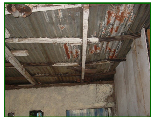
A home in need of a new roof. We get many requests...
